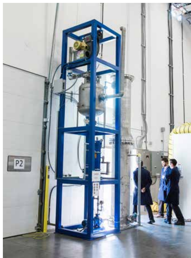
Flue gas conditioning unit at CMCRI's carbon capture and conversion facilities in Vancouver.
