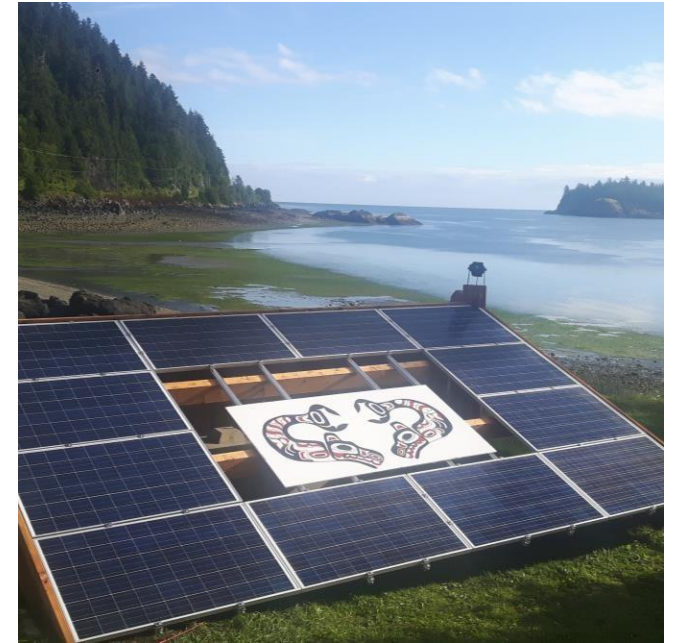
A solar installation at the Haida Heritage Centre helps the Skidegate community move away from diesel and towards energy independence
